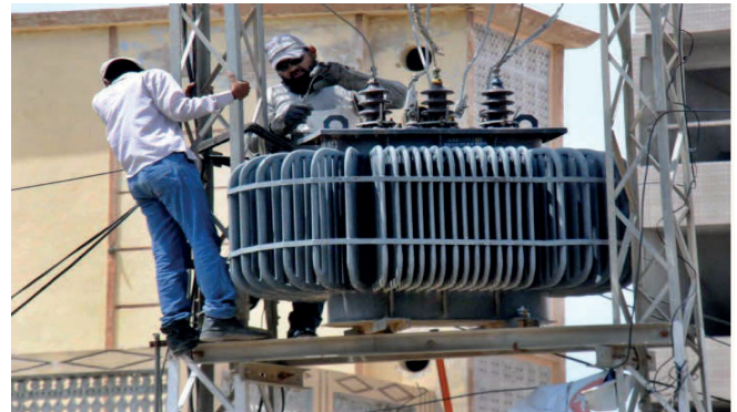
Fig. 1. Pole Mounted Transformers [5].
